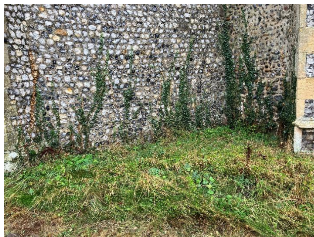
Ivy should be removed to prevent deterioration.
