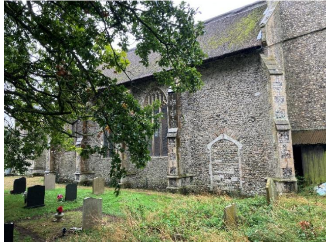
Moss on the thatched roof – ideally would be removed.
