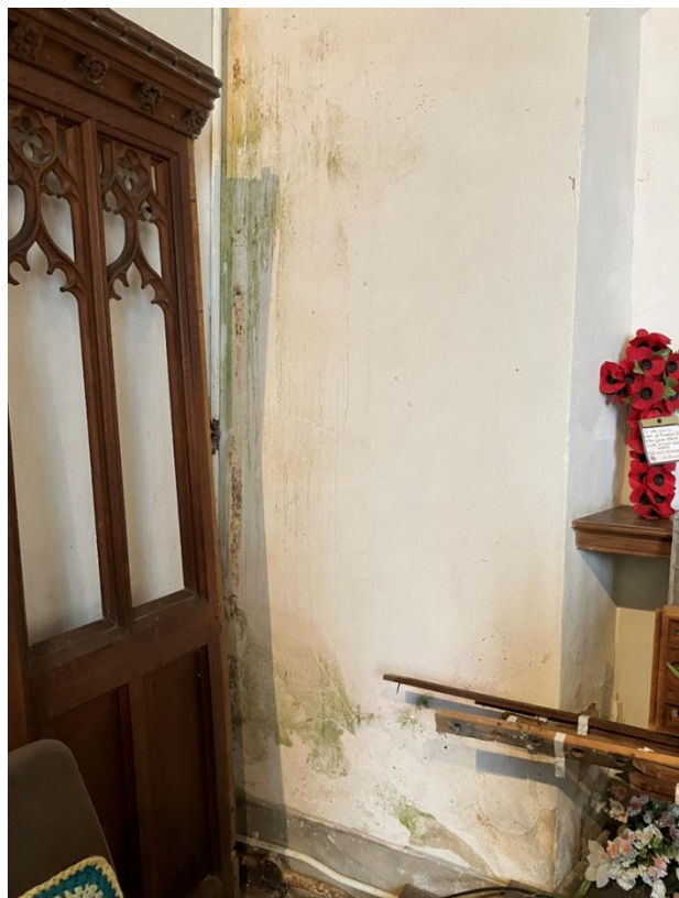
Damp noted on wall adjacent to tower.
