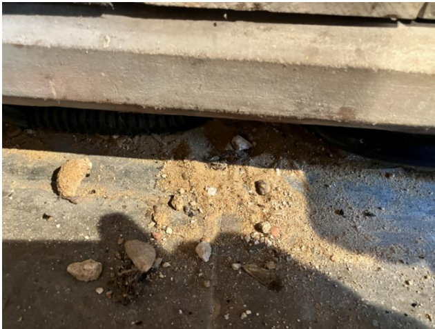
Crumbled base; corner on the left below the north screen.
